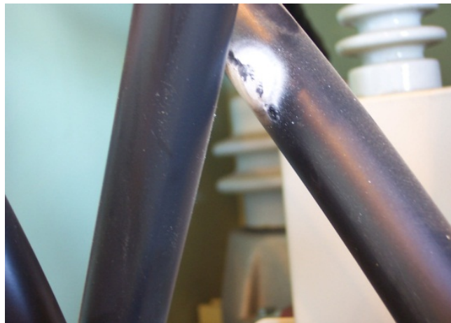
Corona, over time, deteriorated the connection and eventually led to tracking
