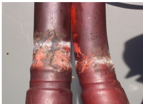
Tracking between two connections led to arcing
