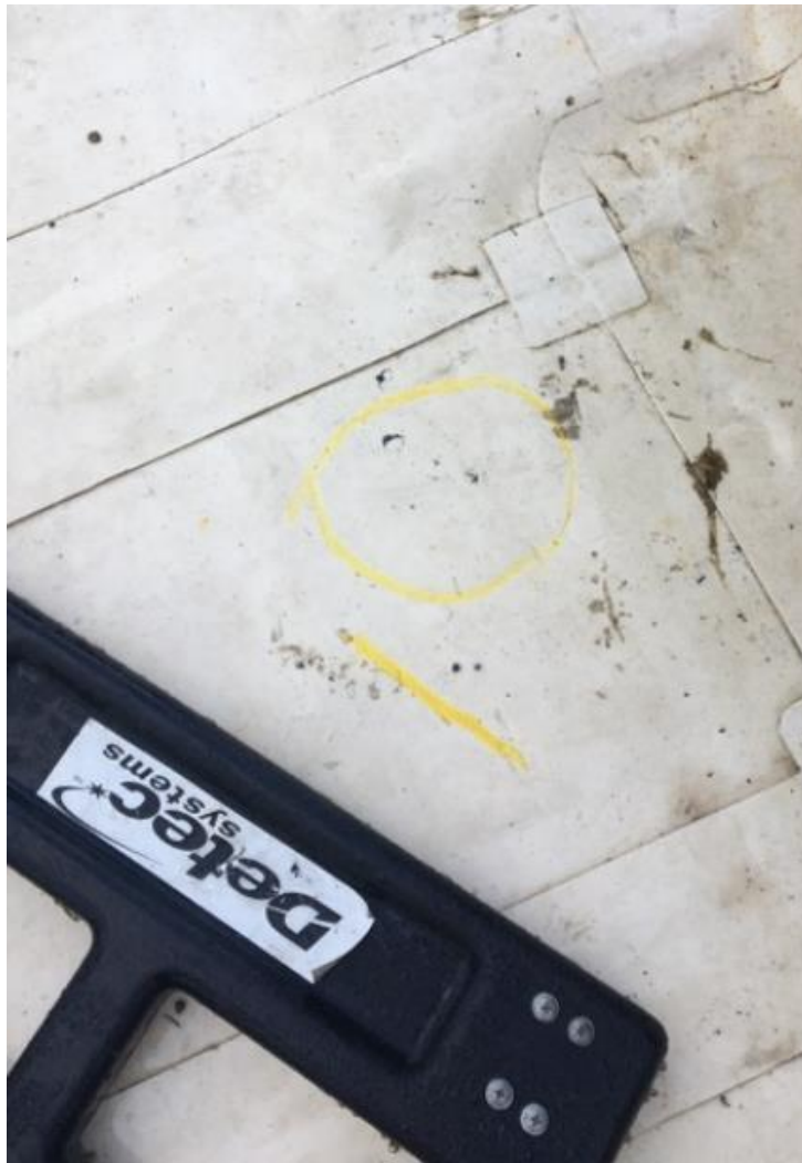
Figure 8: Breach found in a conventional roofing assembly with conductive primer under the membrane.
