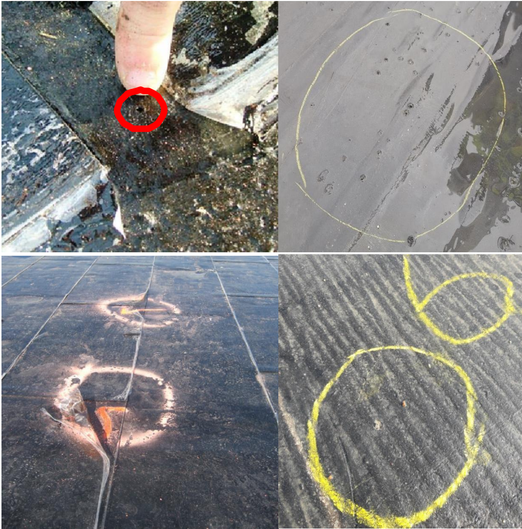
Figure 7: Breaches found in inverted waterproofing/roofing assemblies.
