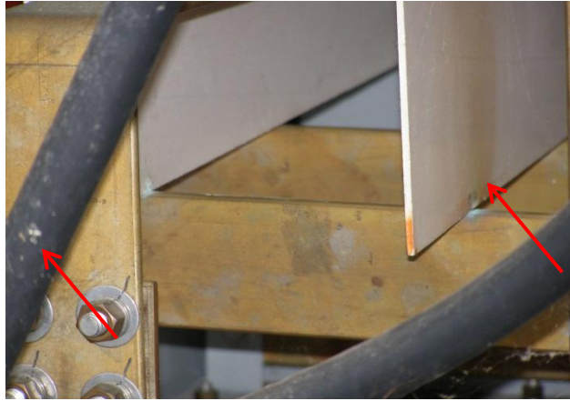
Corona activity advancing to the tracking stage on insulation board resting on 13kV bus. Notice the carbon deposits and light brown discoloration of the insulation board on right.
