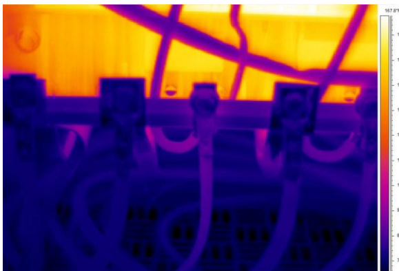
Improper Span and Level using the imager's Auto function.
