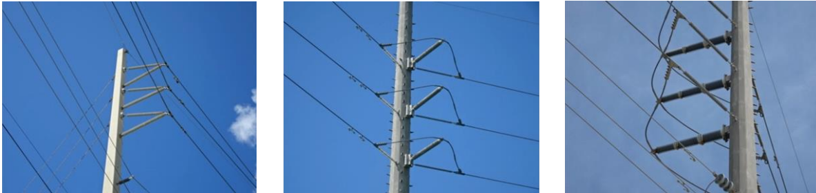
Figure 4: shows typical pole construction of 138kV system with no corona rings. Left image shows 45-degree bracing configuration of polymer insulators, common on most poles. Middle image show a typical dead-end layout using polymer insulators. Right image is a dead-end structure with a mix of ceramic post and polymer dead-ends.
