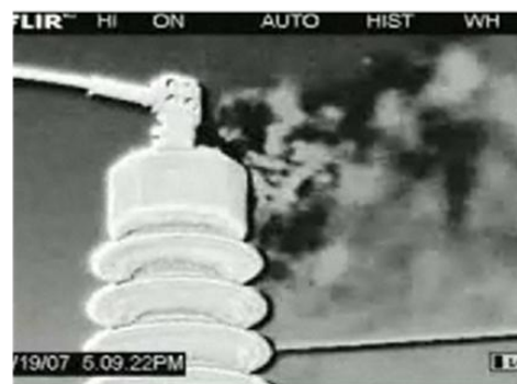
Elec. Circuit Brkr SF6 Leak
