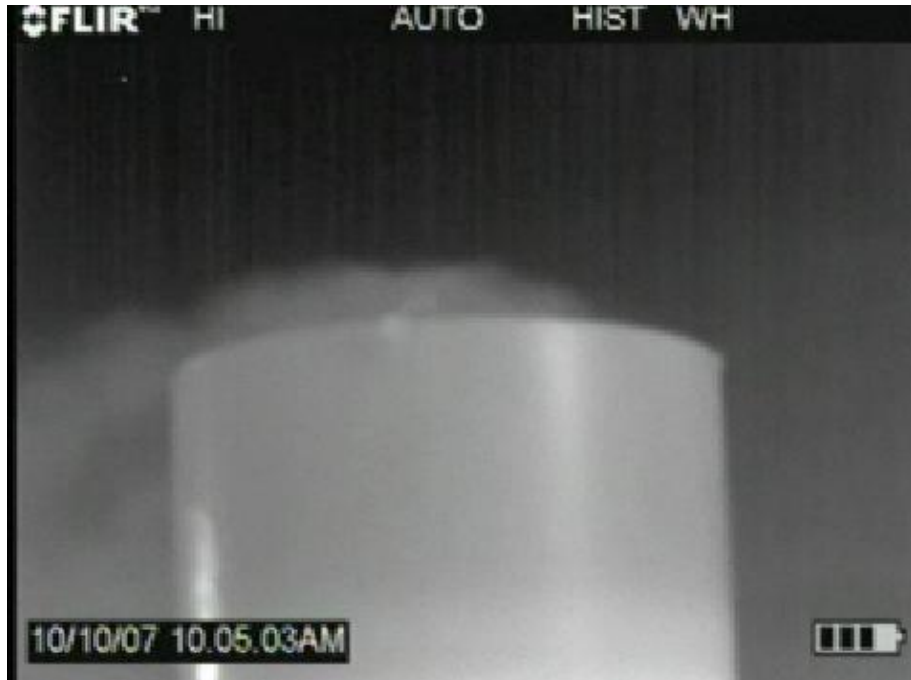
Figure 4. Storage tank leak caused by faulty vent valve
