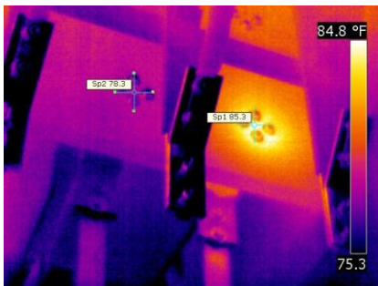
← This image shows the mounting bracket for a stand-off bushing inside a 13kV load interrupter switch cabinet. This insulator is allowing current to leak to ground
