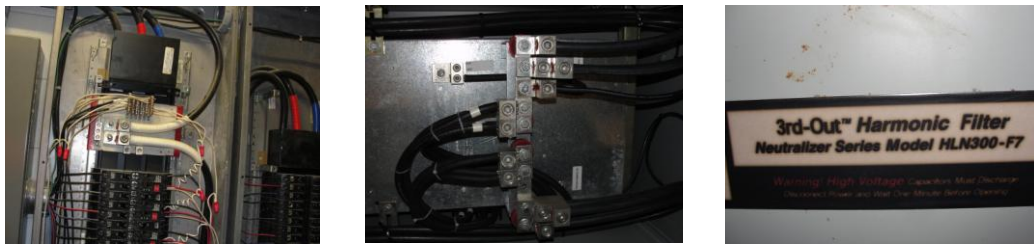
Figure 22a shows an enhanced neutral system in a common 120/208V breaker panel. Figures 22b & 22c are a typical harmonic filter system installed in-line with the main electrical trunk in a data-center facility.
